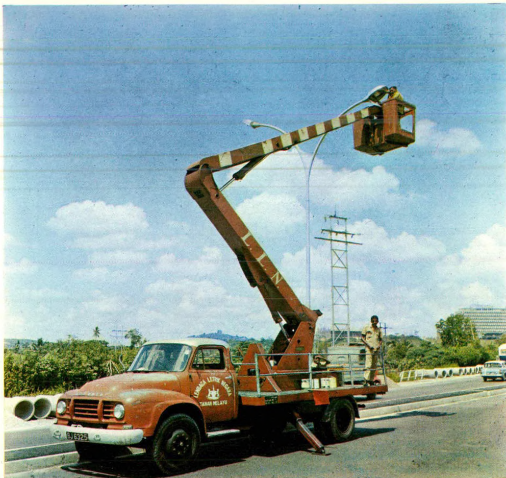
Workmen carrying out street lighting maintenance on a Tower Wagon in Kuala Lumpur, Selangor.
