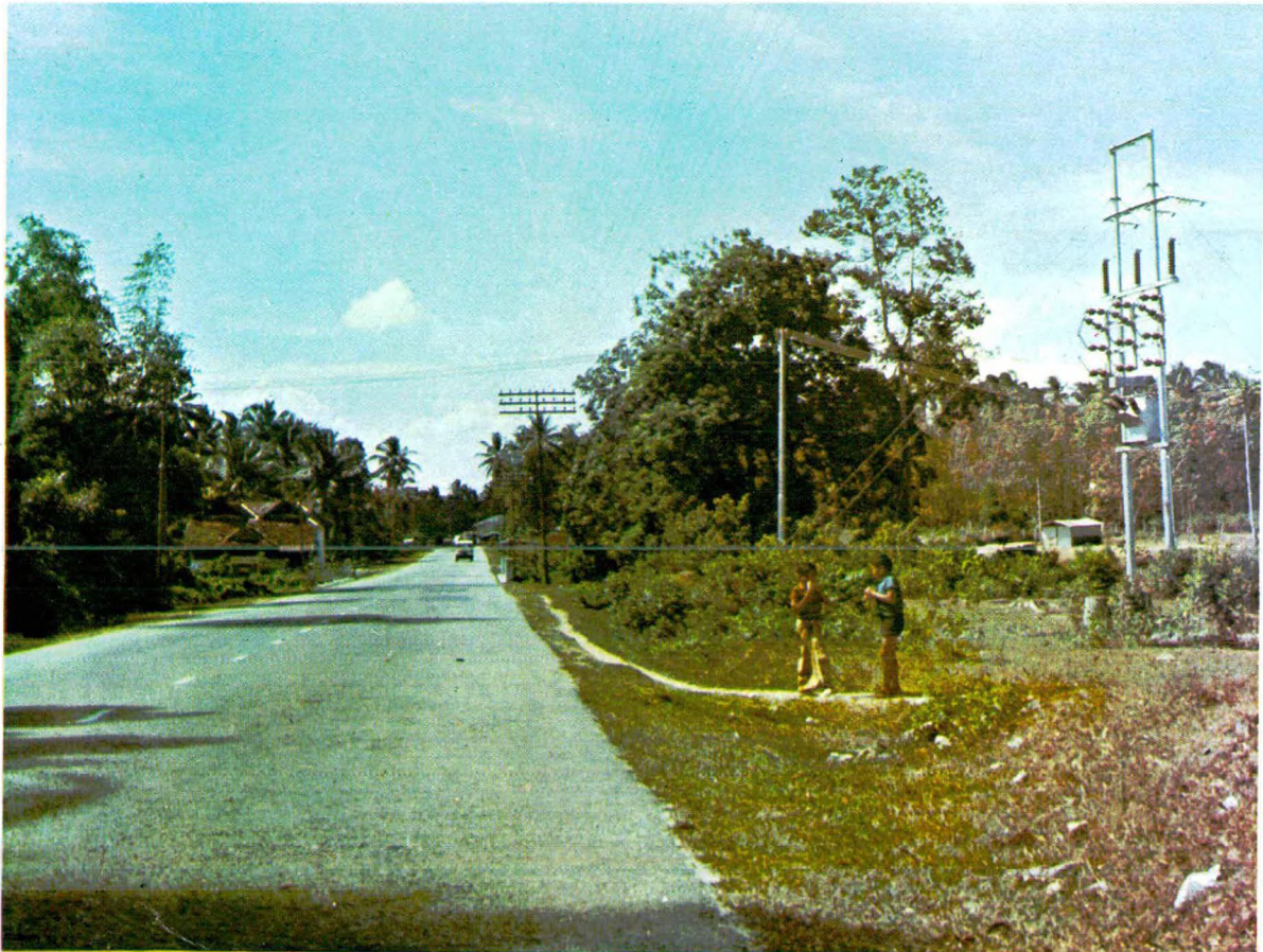
A 33/.433 kV 50 kVA Pole Mounted Substation supplying a Rural Village in Kuantan, Pahang.
